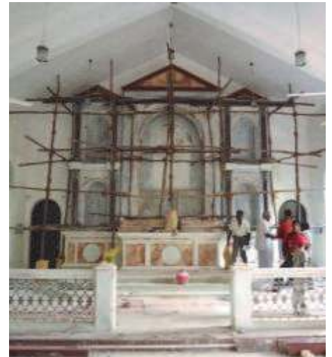
A dramatic baroque altar nears completion at St. Thomas' Chapel, Nagercoil. Marble is relatively inexpensive in India which means that that priestly dreams like this can come true.
