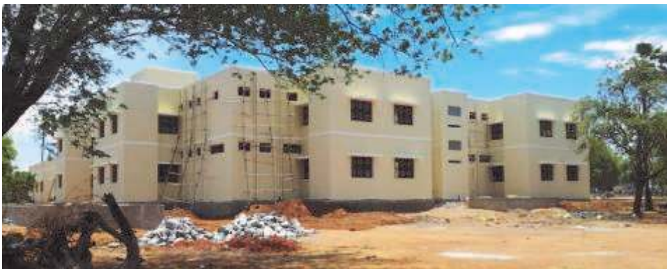
The new 40 room wing of the orphanage is complete after two years of construction.
